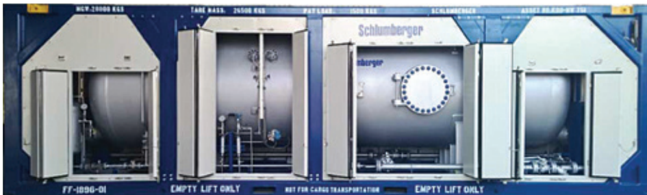
Knockout drum KOD-HW within insulated skid package.
