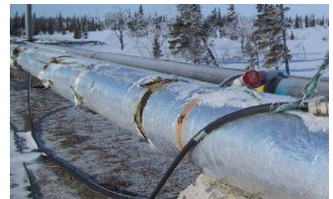
Insulated pipe with electrical heat tracing cable and wool insulation.
